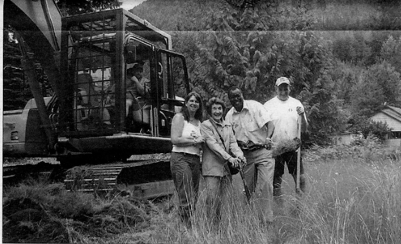
Steelhead Community Association volunteer Paul Roberts sits inside the excavator and watches (left to right) SCA chair Terri Cameron, Steelhead pioneer Doreen Cameron, Mayor James Atebe and project coordinator Roger Pells break ground for the new community hall.
